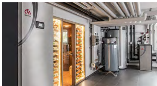
Connection to DHW storage tank, buffer tank and with „free cooling“. The heat pump is connected to geothermal probes.
